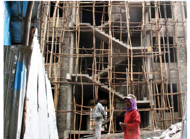
At this future wing of a city hospital, six female laborers work alongside some 60 men.
