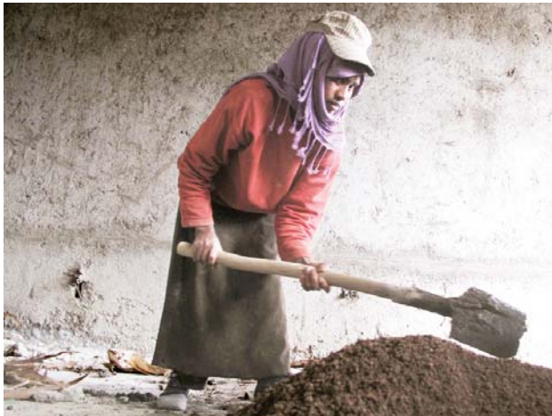
Mekedes Getachew, 19, has been working at construction sites in Addis Ababa, Ethiopia, since she was 15 years old. Except for the heaviest lifting, she says, the laborers "all do the same work and we don't really say this is a man's job, but when it comes to salary there's a difference." She earns $1.50 a day. Men earn $2. Photo Credit: Gregory Warner/NPR
